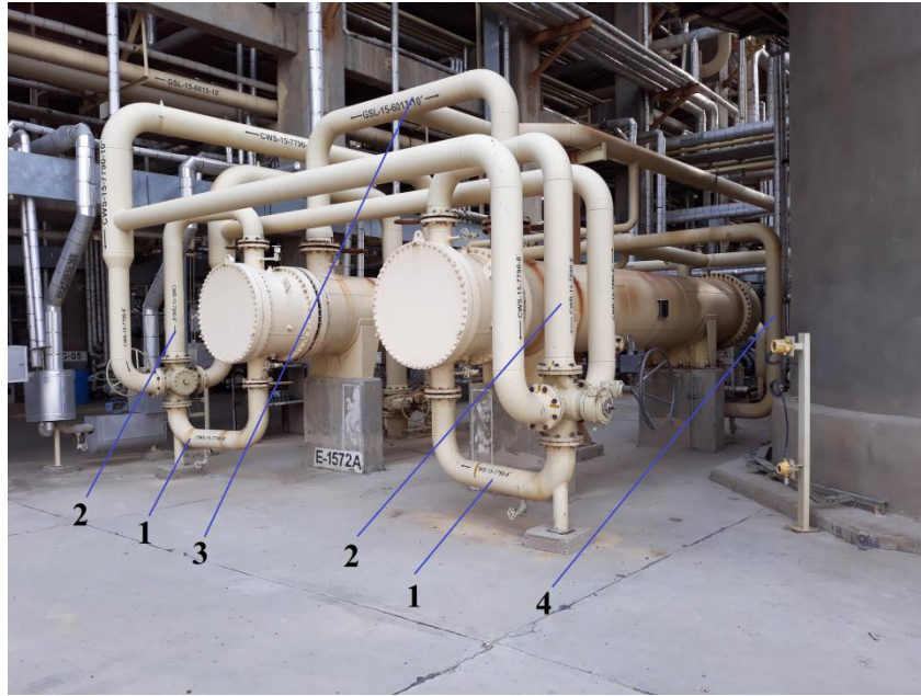
Fig.1. Real shell and tube cooling heat exchangers of the RFCC gasoline product that have been modeled. (1) Inlet cooling water to tubes, (2) Outlet cooling water from tubes, (3) Inlet gasoline product to shell, (4) Outlet gasoline product from shell
